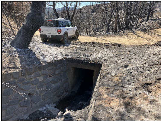
Picture 8. Box culvert at Hummingbird Creek on San Dimas Experimental Forest (USDA FS)
