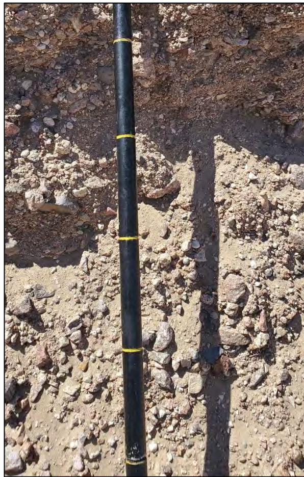
Figure 9. Lamego Ditch Bridge west wall on the north side of the bridge
