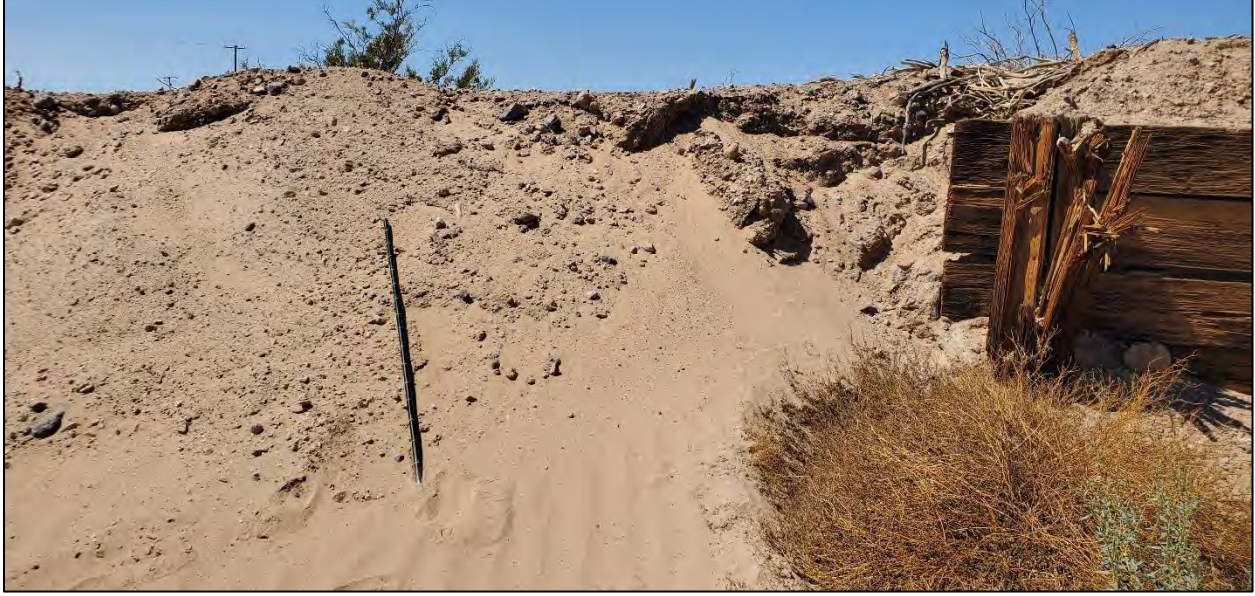
Figure 8. Lamego Ditch Bridge west wall on the south side of the bridge
